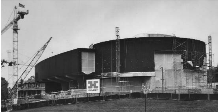
Miller & Long's work on the American University Katzen Arts Center in Washington, D.C. included careful pours for the building's exposed concrete walls and floors.
